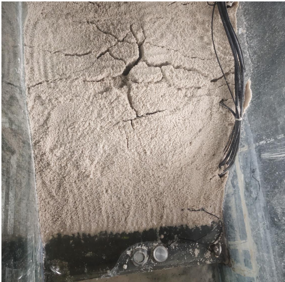
Figure 4-4: Did not fail only seepage and crack ground water 16cm.
